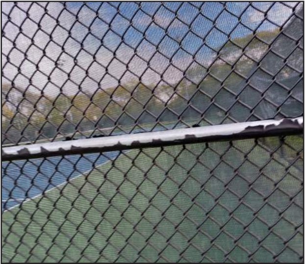
Tennis court fencing condition
